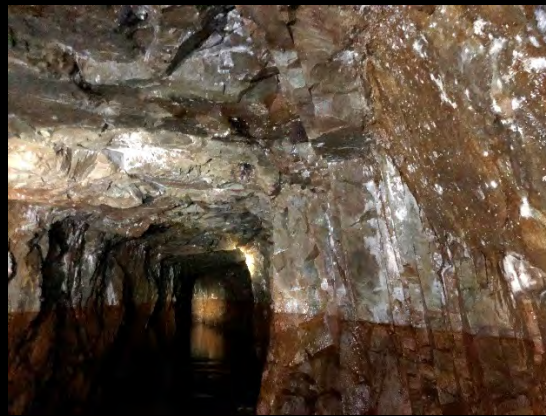
ca. 600 m; open tunnel. Water mark at ca. 160 cm water depth. Wet ceiling
